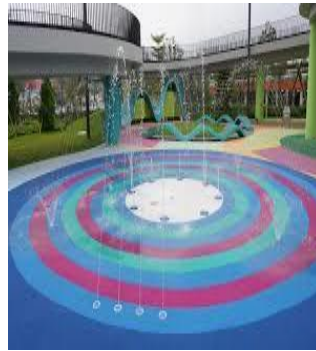
Water Feature System at KTSP
